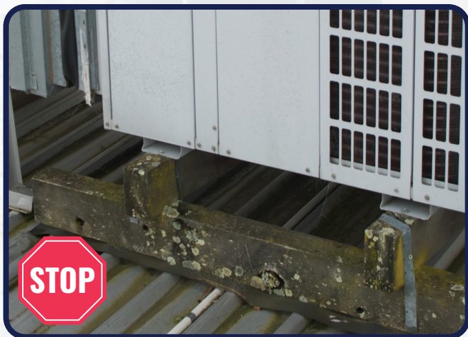
(HVAC fixed with wooden dunnage)
